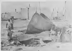
These heavy steel mats protect against the "throw" of rocks and debris. In the foreground some of the 1600 holes are loaded with explosives.
